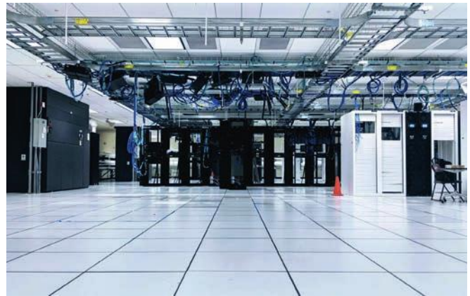
■ A server room
