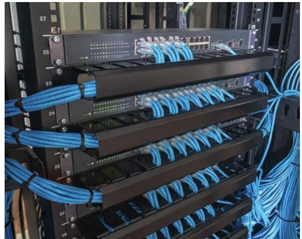
■ Network switch and ethernet cables
